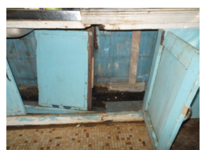
This sink bench and the cupboards in student kitchen needed urgent work. An Australian Mission's Work Team is here to help tidy up.
